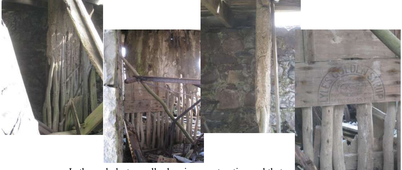
Lathe and plaster walls showing construction and that all spare timber was used.
