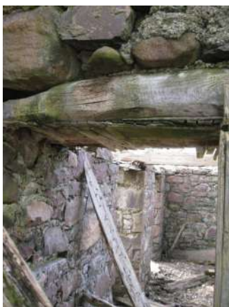
Looking into S. room with wooden lintel and line of additional wall
