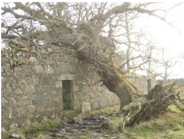
Remains of the rear wall at risk!
